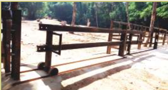
Railing of Indian Elephant Enclosure: A new barricade was constructed at Indian elephant enclosure using heavy gauge iron railings.
